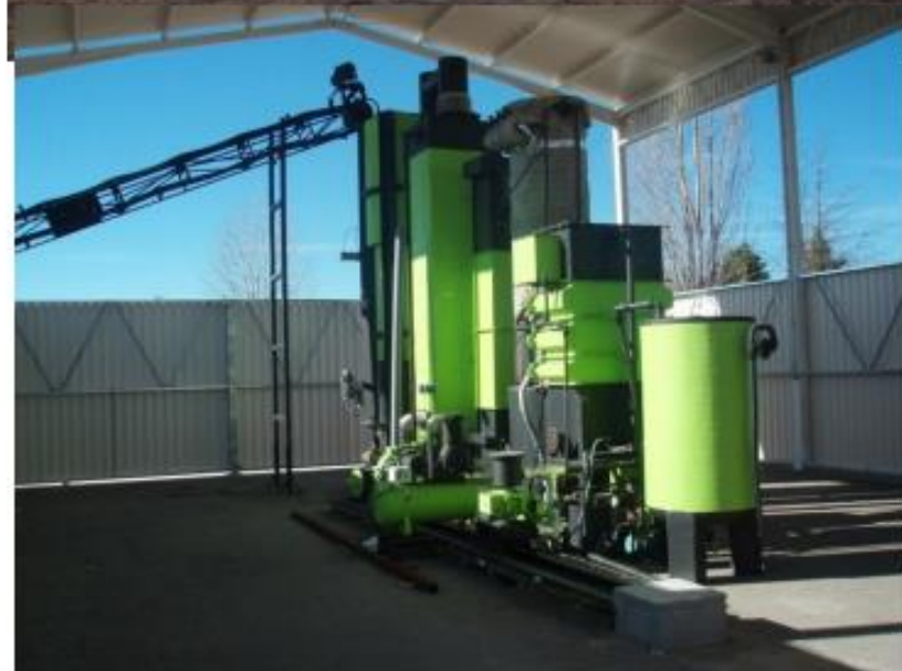
50kg/h R&D BIOMASS GASIFICATION PLANT
